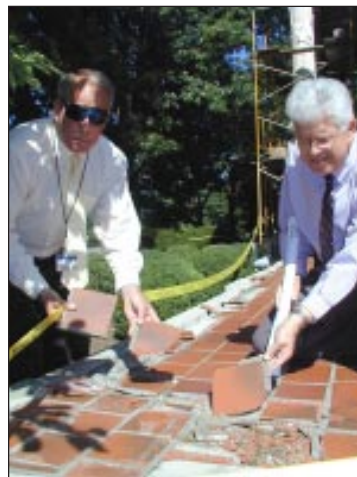
General Services Acting Director David Pentz (l) and Acting Deputy Director Bill Pauley display areas that need to be repaired at the Governor's Mansion.
