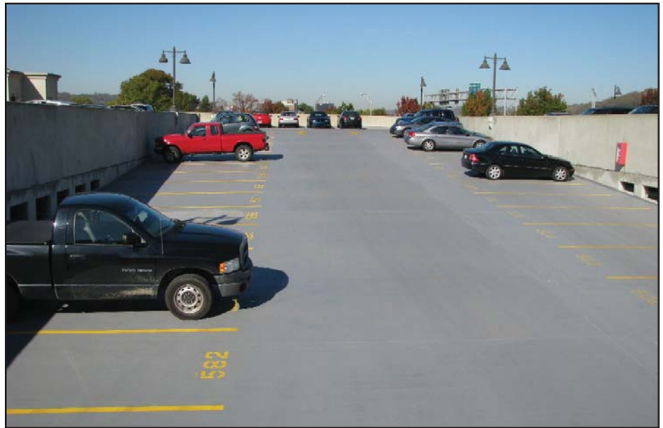
Concrete repairs and repainting of parking lines are among the fixes made to the Capitol Parking Building. The building repairs are expected to be done in December, ahead of schedule.
