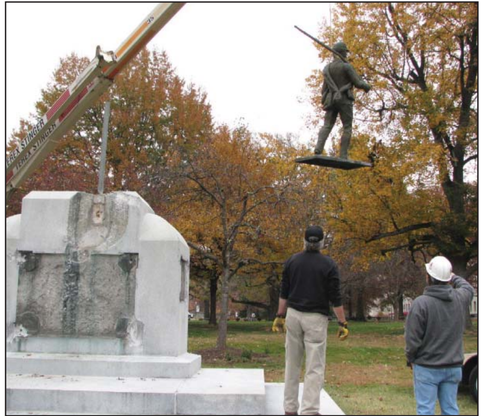
The Soldiers and Sailors Monument will return to its perch on the south side of the Capitol lawn once the restoration project is complete. The cracked granite foundation underneath the statue is being replaced and the four plaques and Union soldier figure will be cleaned and restored to their original finish.
