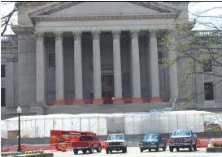
Renovations made to the North Portico of the main Capitol Building is an example of the work being done at the Capitol Complex.
