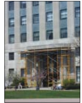
Above: An inspection of the entrance of Building 3 is currently taking place due to loose limestone which has fallen.
