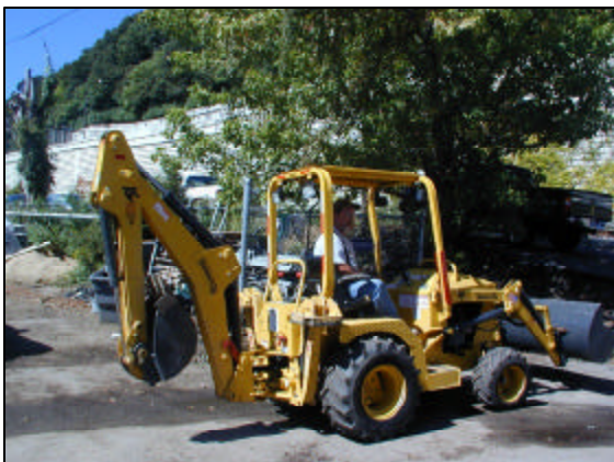
General Services' Billy Tincher worked this Teramite backhoe until 10:30pm at night correcting a drain problem near a data vault as a result of Hurricane Frances.
