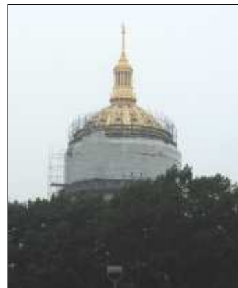
The white covering that has allowed work to continue through various weather conditions began coming down in early September.
